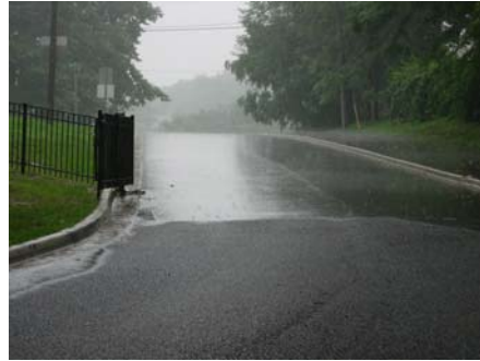
Porous asphalt during a rain storm at the entrance of Willard Beach in Battle Creek
